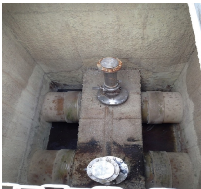
Figure 1. Concrete Deterioration in Sanitary Sewer Structures due to MIC
