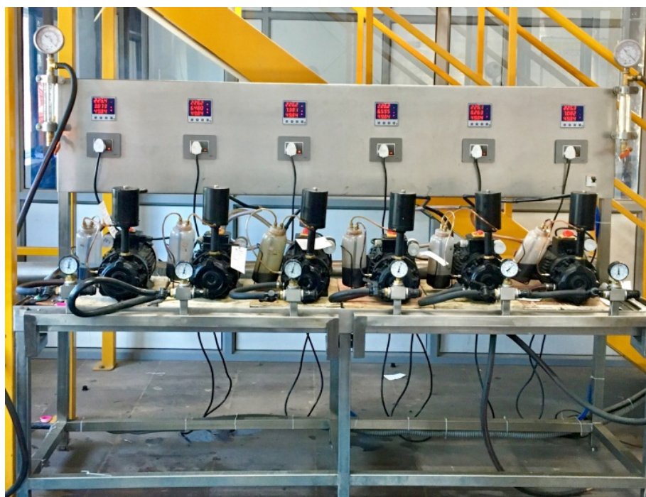
Figure6. Vacuum Pump Testing Setup
