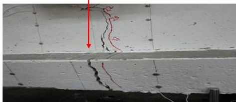
Figure 5: Failure mode of beam B5
