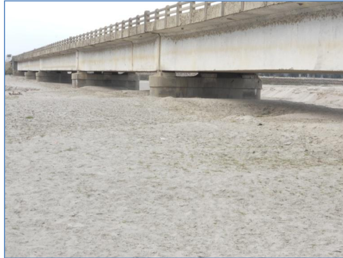
Plate 1- Siltation below of Jiadhoh RCC Bridge at N
