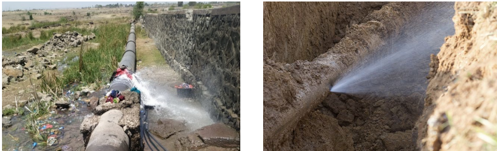
Figure No. 1 Visible and Non-Visible Leakages
