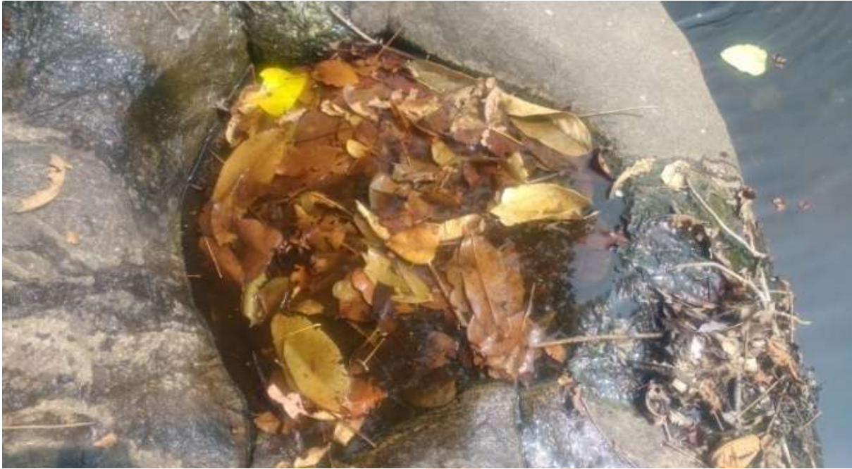
Figure 1: Leaf choked pothole
